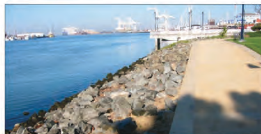
► Figure 3.9.g: Riprap is not accessible.
