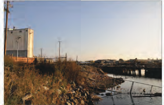
Figure 3.8.a: Neglected cyclone fencing along the Estuary frontage.
