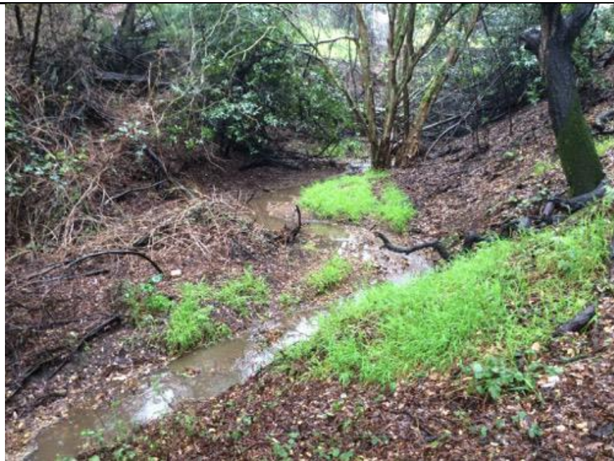
Photograph 3: Culvert outlet at the end of Sage Road. Photograph taken on January 14, 2015.
