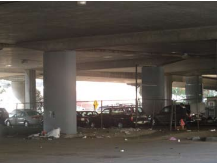
Trash accumulates under the freeway is an eyesore for the community.
