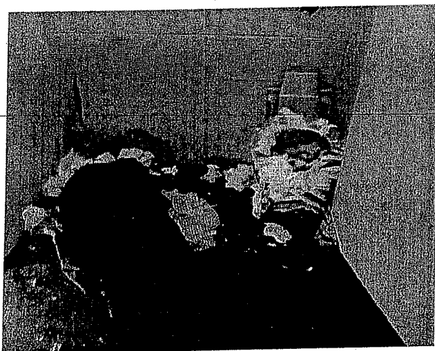
District 7: Officer Willie Wilkins Park restroom stall
