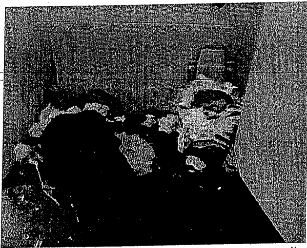
District 7: Officer Willie Wilkins Park restroom stall
